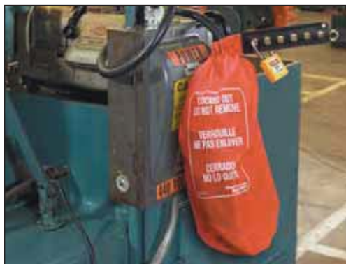
Electrical Connector Lockout
